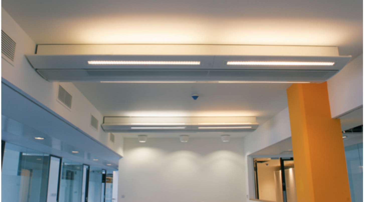
Chilled ceiling in Kings College
