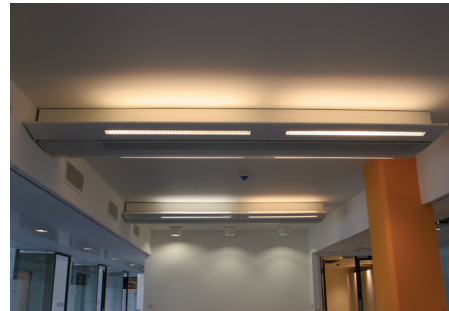
As part of a sustainable solution for the refurbishment of the Strand Building of King's College London, nearly a kilometre of active chilled beams with integrated lighting have been installed.
