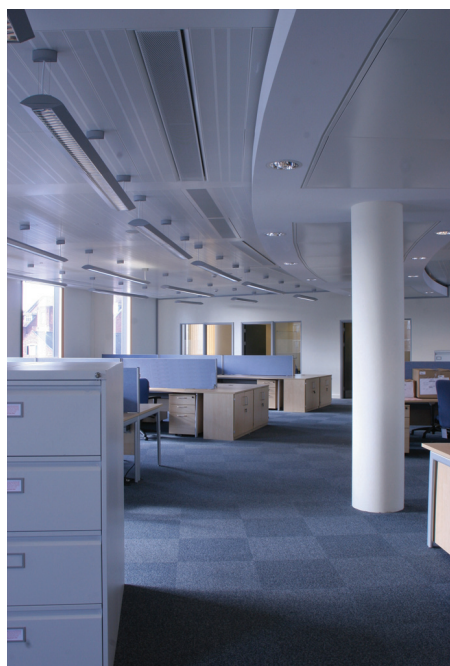
To help achieve the highest possible BREEAM rating for the recently opened Jobcentre Plus in Bournemouth, cooling and fresh air are provided by SAS active chilled beams.
